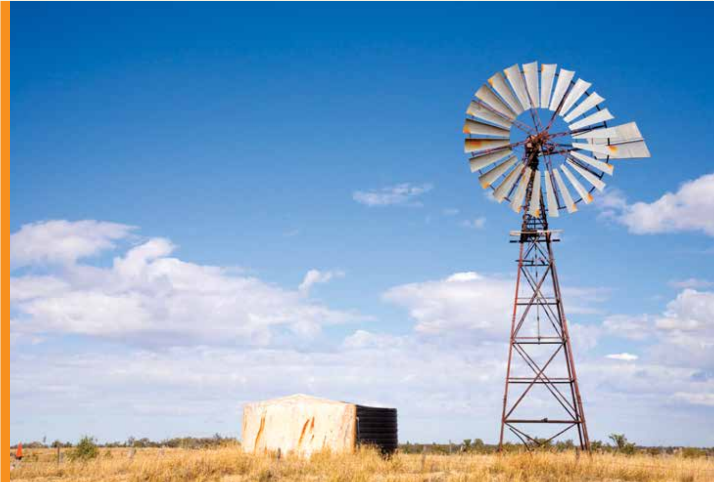
Figure 21 – Typical farm bore installation
