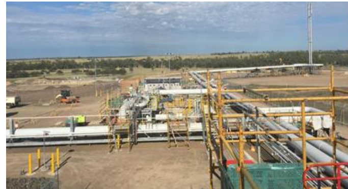
Charlie Field Compression Station – view from side
