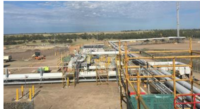
Charlie Field Compression Station – view from side
